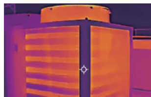
HVAC Leak Detection
