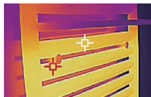
HVAC Leak Detection
