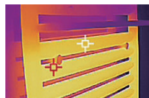
HVAC Leak Detection
