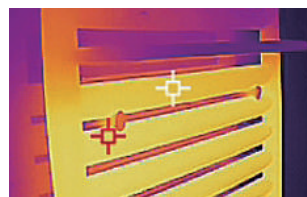
HVAC Leak Detection
