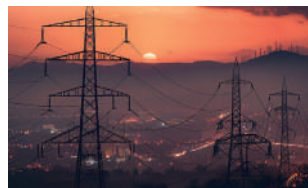
Electric Routine Inspection
