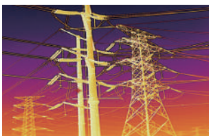
Electric Routine Inspection
