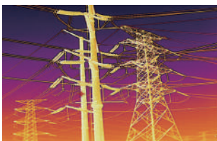
Electric Routine Inspection
